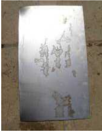
Picture 9: Back plate of combustion chamber
