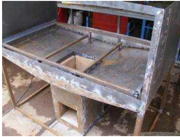
Picture 54: Image of baffle square pipe supports attached
