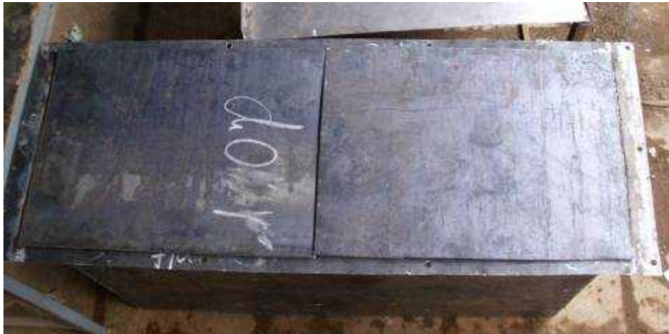
Picture 43: Doors in combustion chamber
