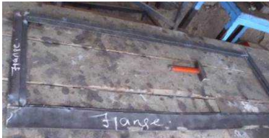
Picture 27: Oven chamber flange on top of baking chamber flange
