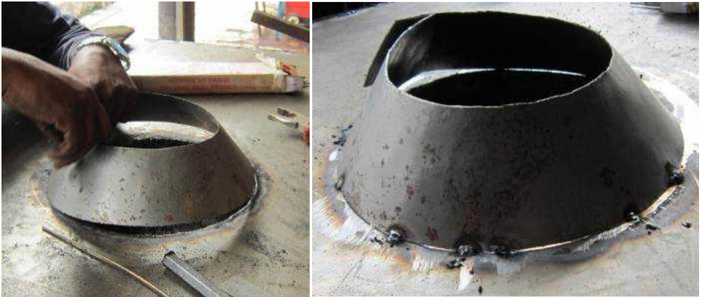
Picture 67: Images of manifold shaped to fit hole (left) photo of manifold spot welded on with excess material (right)
